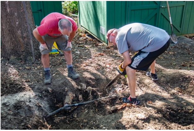
A water pipe ran through the project site, along with many roots. Mr. McGrath and Mr. Stroh working to remove the roots.
