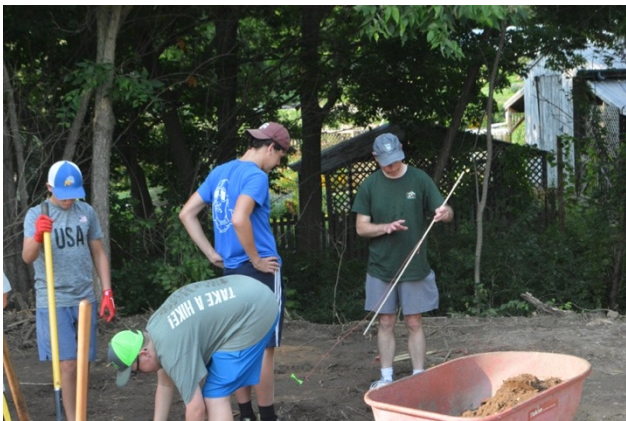
Mr. Lohmueller explaining to Nick Stroh a technique to determine if the foundation is level
