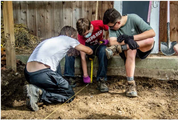
Isaac Lohmueller, Petey Wilkens, and Wesley Anglin checking if the work site is deep enough
