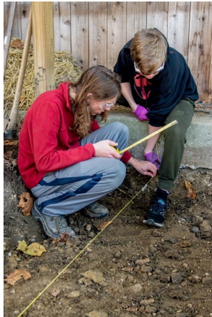
Isaac Lohmueller and Petey Wilkens checking if the work site is deep enough
