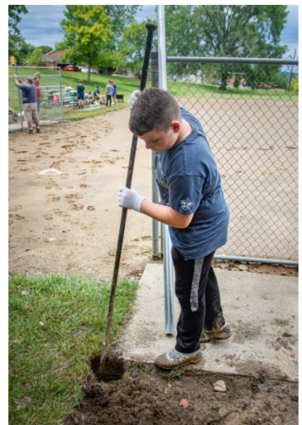
Travis Anglin breaking up a rock in the bottom of a fence post hole
