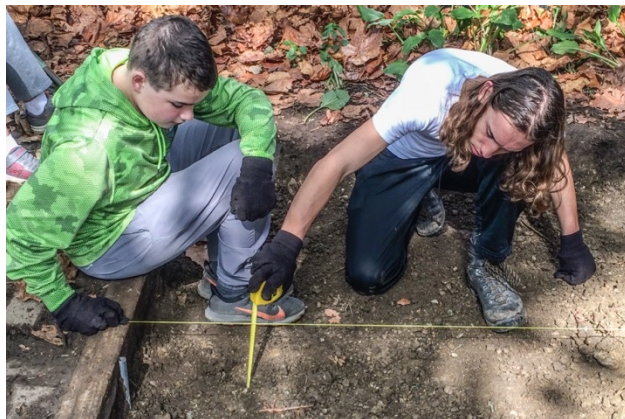
Travis Anglin and Isaac Lohmueller checking the depth of the patio foundation
