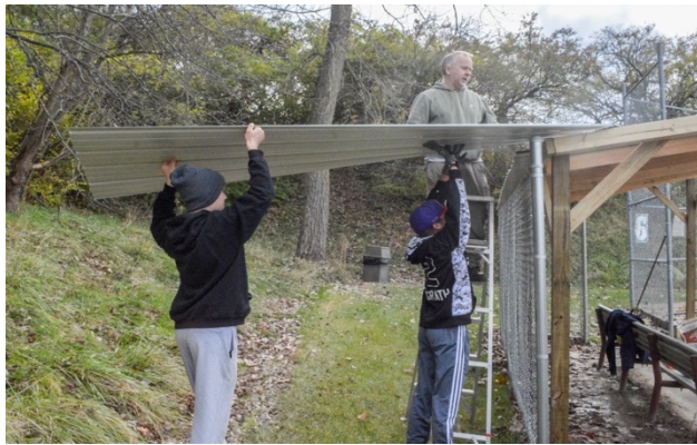
Petey Wilkens and Declan McGrath lifting a piece of the metal roofing
