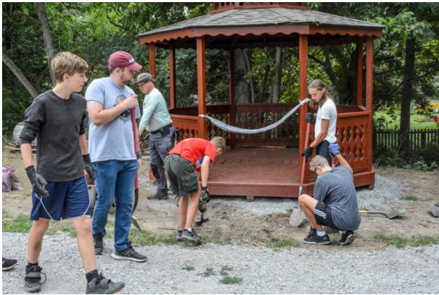
The team started to dig out the foundation for a paver walkway up to the gazebo
