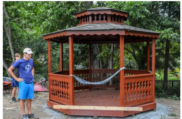
Once the gazebo was positioned, Nick Stroh made some repairs and painted the wood
