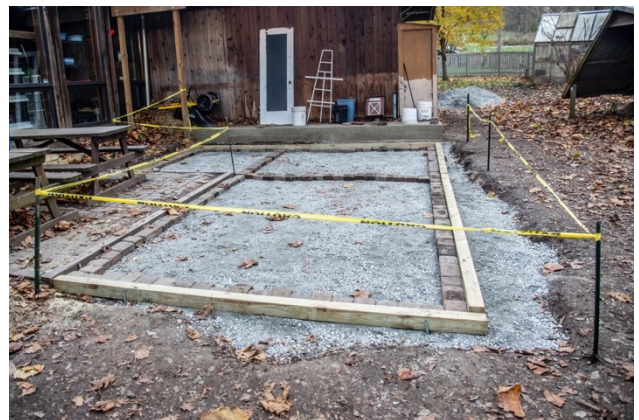
The end of another workday. The bricks were laid out on the perimeter of the patio to check alignment of the bricks.
