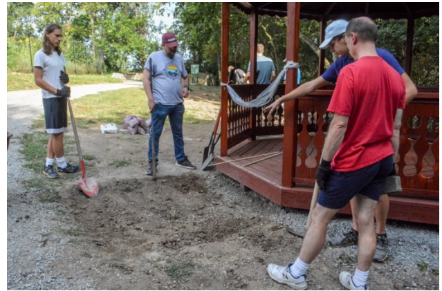
Nick Stroh and Mr. Lohmueller discussing how to tackle the walkway construction
