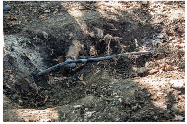
A water pipe ran through the project site
