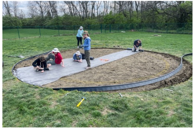
Several scouts started to lay the landscape fabric while several others were finishing up the border
