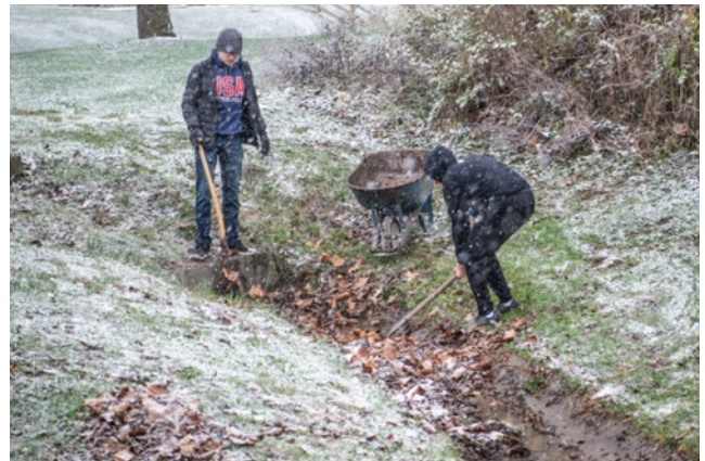
The drainpipe for the ravine was plugged with dead leaves. Petey Wilkens and Nathan Hoffman
