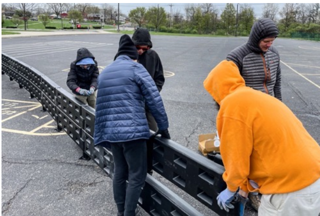
Assembling the wall. It turned out to be very difficult to get the wall together. The pieces did not fit well, so the scouts were sitting on it and holding it at different angles to try to get the posts in correctly. This took much longer than expected.
