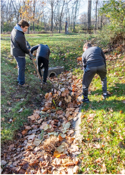
The end of the drainage ravine had a lot of dirt buildup
