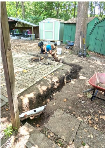
Petey Wilkens had to dig a trench from the main building to the shed for an electrician to run wiring
