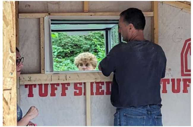
Working to install the AC unit in the wall of the shed.
