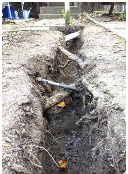
The trench had to be dug around roots, a drainpipe, and a water line
