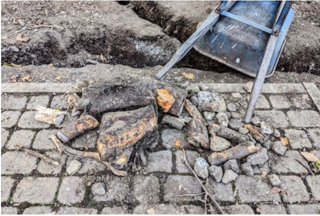
Some of the root and rock obstacles that had to be overcome while digging the ditch for the electricity
