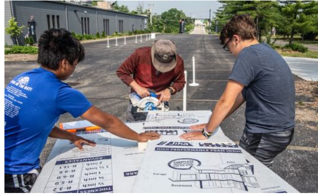
Mr. Wilkens cutting the insulation sheets while one of Pety Wilkens' friends and Nathan Hoffman hold the panel
