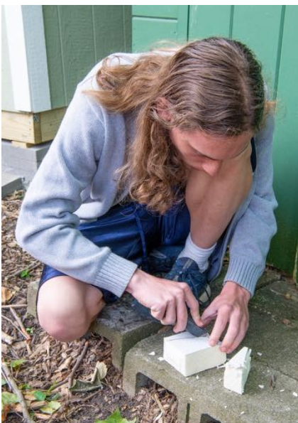
Isaac Lohmueller cutting the insulation to fit into the gaps around the door
